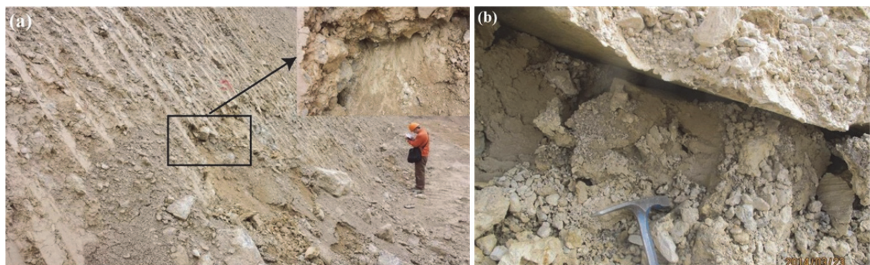
Fig. 2 Deformation conditions of the Tangba earth quarry slope in Mar. 2014. (a) Shear outlets at the elevation of 2,120.0 m; (b) Shear outlets at the elevation of 2,210.0 m.
