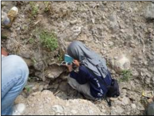
Figure 3 Bedrock of jointed andesitic breccia covered by the weathered material of sandy clay (exposed at the foot of susceptible mountain slope). Contact between the breccia and sandy clay performs as the sliding surface.
